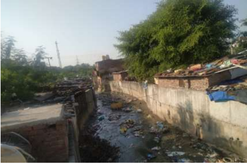
A view of Drain passing though a slum in Jammu
